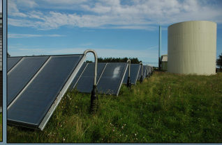
Solar plant for heat grid
